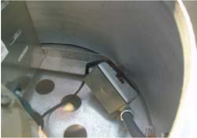
Picture 1: EFH1's Disconnect Switch
