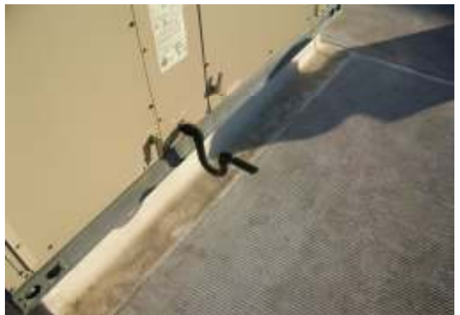
Picture 6: Drain Lines Properly Installed
